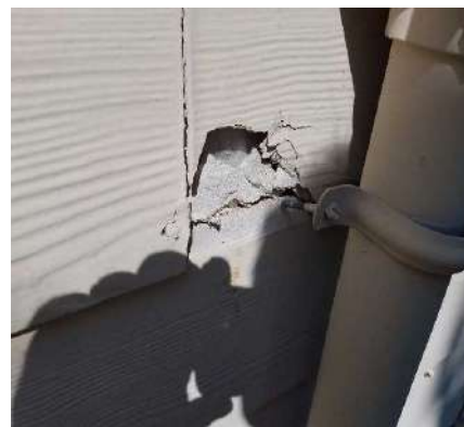
Near Electric Utility Entrance
